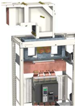
Direct connection of the Canalis KT busbar trunking on the Masterpact 3200 A circuit breaker.
