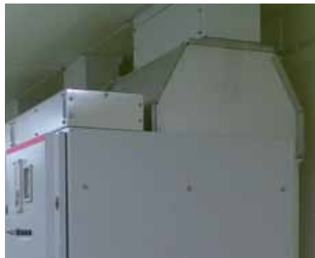
Figure 59: Example of switchgear with gas duct with outlet (total height of the switch-gear is 2675 mm for 12-17,5 kV up to 40 kA)
