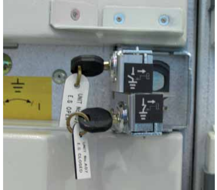
Figure 6: Double key lock on earthing switch
